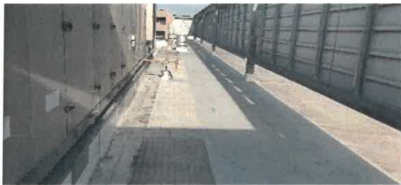
Photo #3 Overview of the center section of one of the roof sections inside the equipment screen wall.
